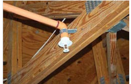
Residential fire protection sprinkler head
