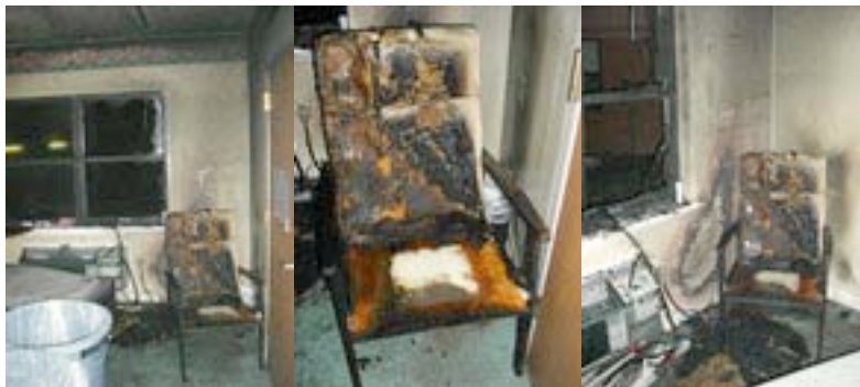
The Difference a Fire Sprinkler Makes...
